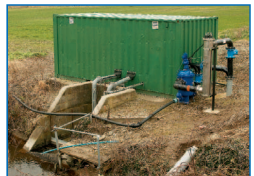
TOP. Field of organically grown spinach. CENTRE. Boll 6.18 Automatic Filter. ABOVE. Packaged filtration and UV treatment plant for purifying river water used for crop irrigation installed at Abbey Farm.
